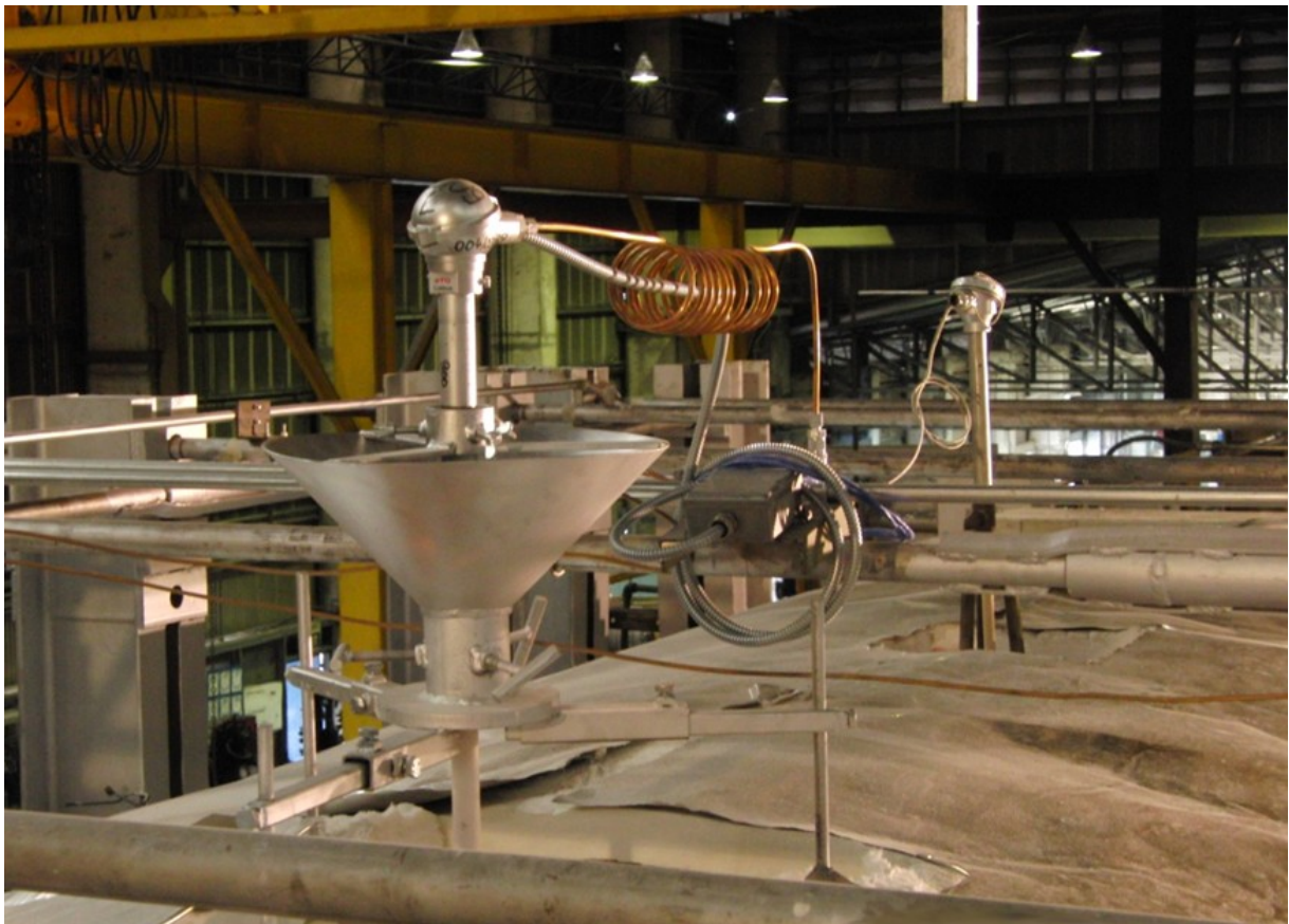
Picture I: Oxygen sensor in regenerator crown installation
